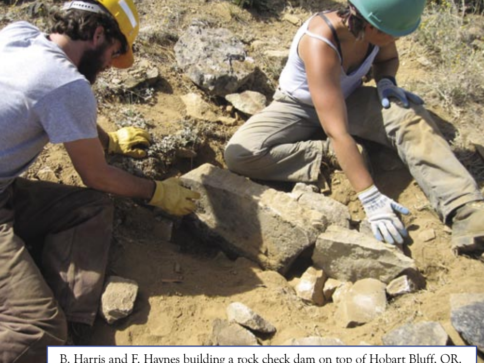
B. Harris and F. Haynes building a rock check dam on top of Hobart Bluff, OR.
