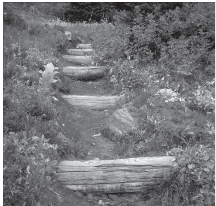
Figure 1. Large check dams, over the years, will help this gully fill in. These check dams need an apron of loose rocks down from each log to prevent water scouring. Scarifying, planting rocks and transplants, adding fill, seeds, and debris will speed the process. (IMAGE COURTESY OF THE USFS)
